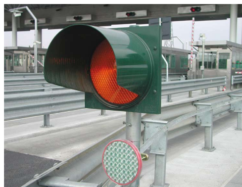
Flashing device on highway application
