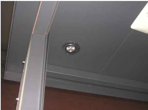
Internal lighting ceiling spotlight
