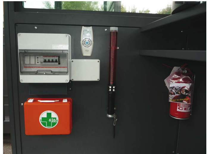
Electrical panel, first-aid kit, luminous sticks multifunction, fire extinguisher
